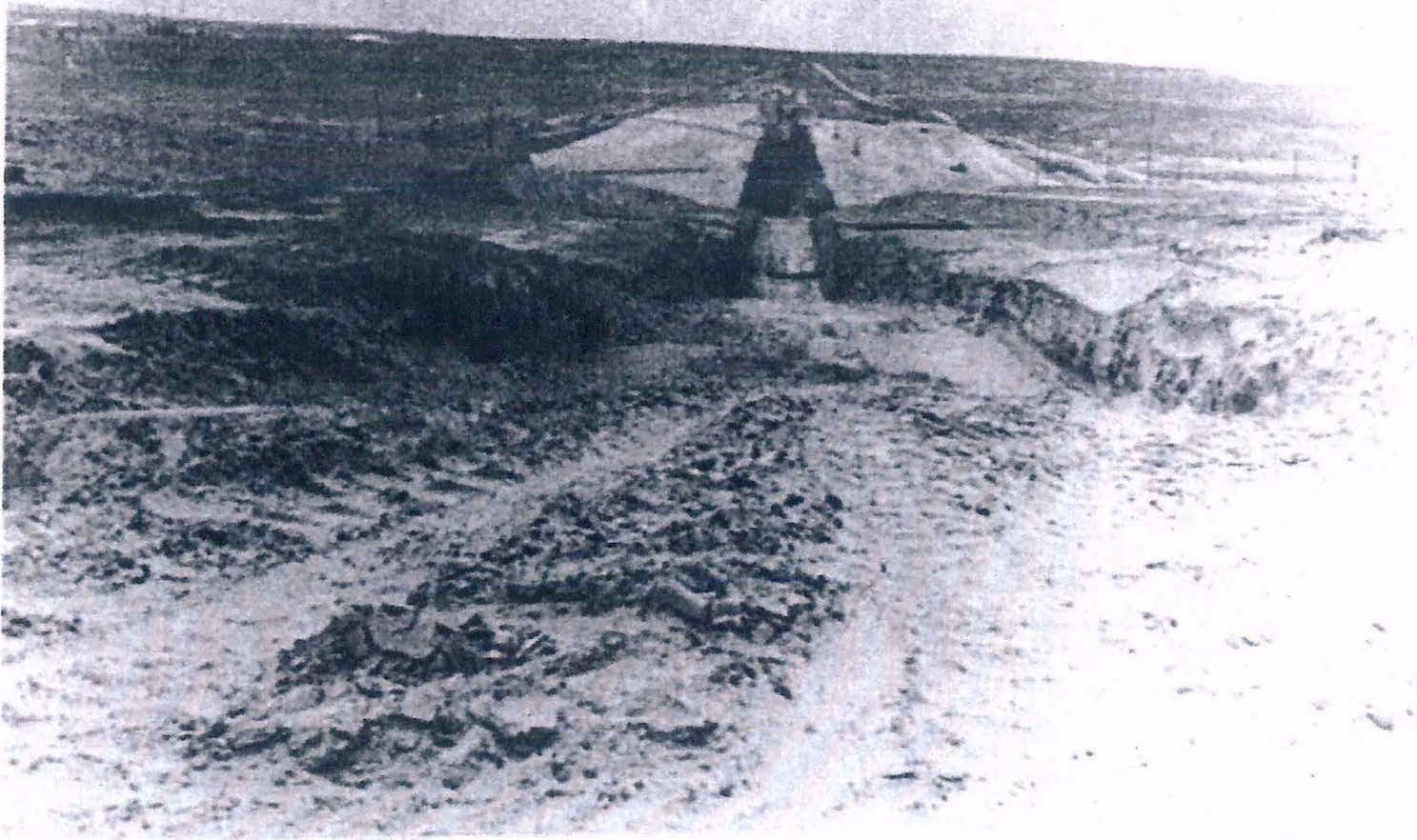
Excavation for Morgan Lake Dam. To the right of the cut (East) will become Morgan Lake. 5/17/61
